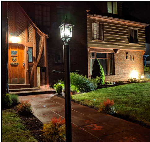
Some results of the lighting project.
